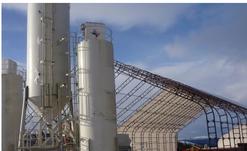
On-site paste plant for use underground
