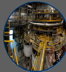
Concentrate Thickening & Filtration
